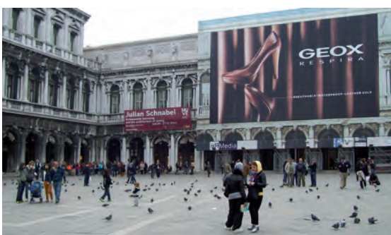
© Alena Sobotova - Advertising on the restoration worksite of the Ala Napoleonica facade in St. Mark's Square
